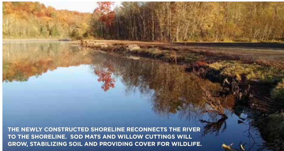
CONSTRUCTING COARSE WOOD SHORELINE STRUCTURES THAT PROVIDE HABITAT PROTECTED FROM RIVER FLOW AND PREDATORS.
