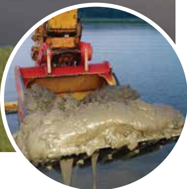
NATURAL REVEGETATION WILL CREATE EXCELLENT HABITAT FOR FISH. BELOW: THIS IS THE LAST BUCKET OF SLUDGE.
